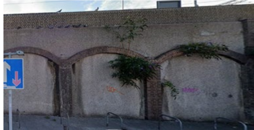
Existing arches at Courtenay Place are closed up, with poor quality public realm and unused cycle stands
