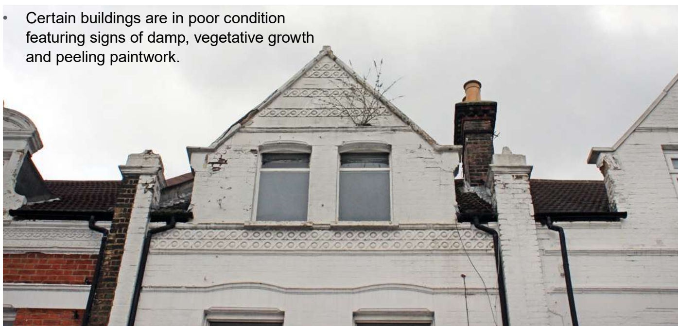
A gable in disrepair and showing signs of water ingress and vegetative growth
