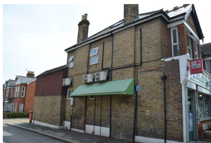
Face fixed plant and cabling
