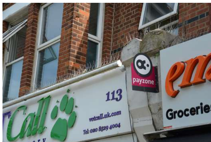
Pigeon deterrent spikes
