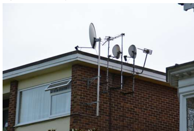
Satellite dishes and aerials
