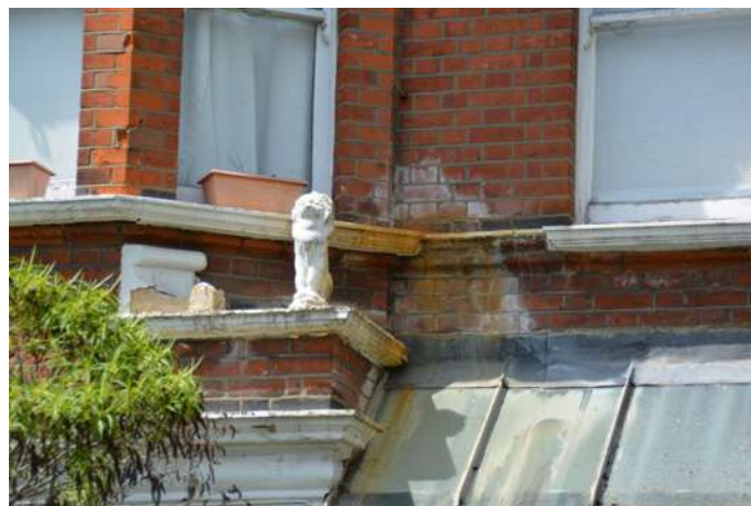
Lack of effective maintenance.
