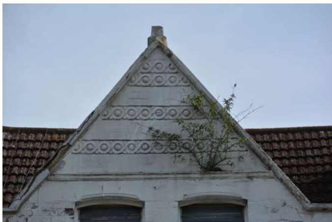
Overall state of disrepair to certain properties.
