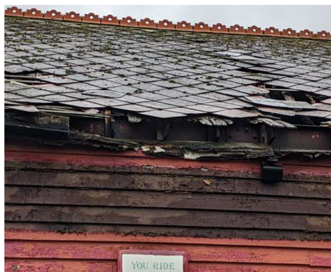
Rotten timbers and slipped roof tiles at the Queen Elizabeth Riding Stables
